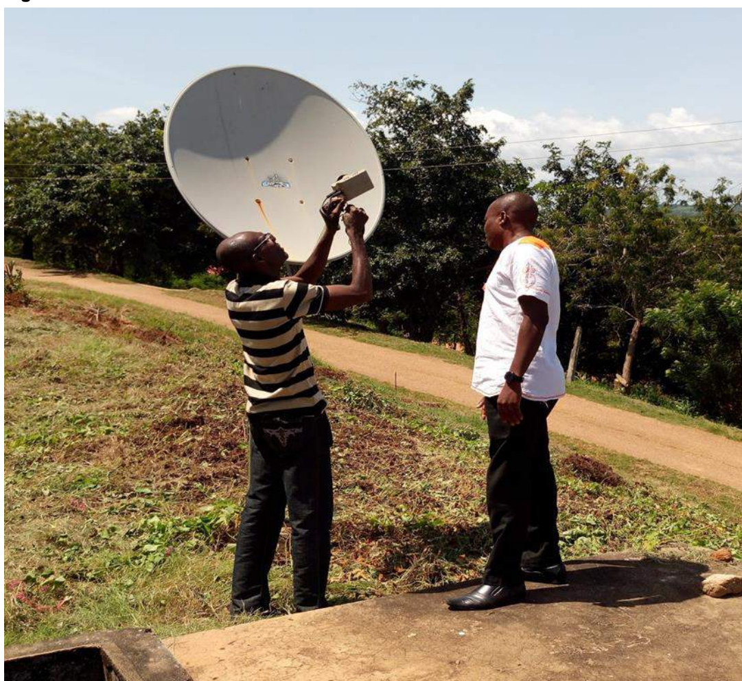
Figure 12: Komenda CoE ISP Connection Point
